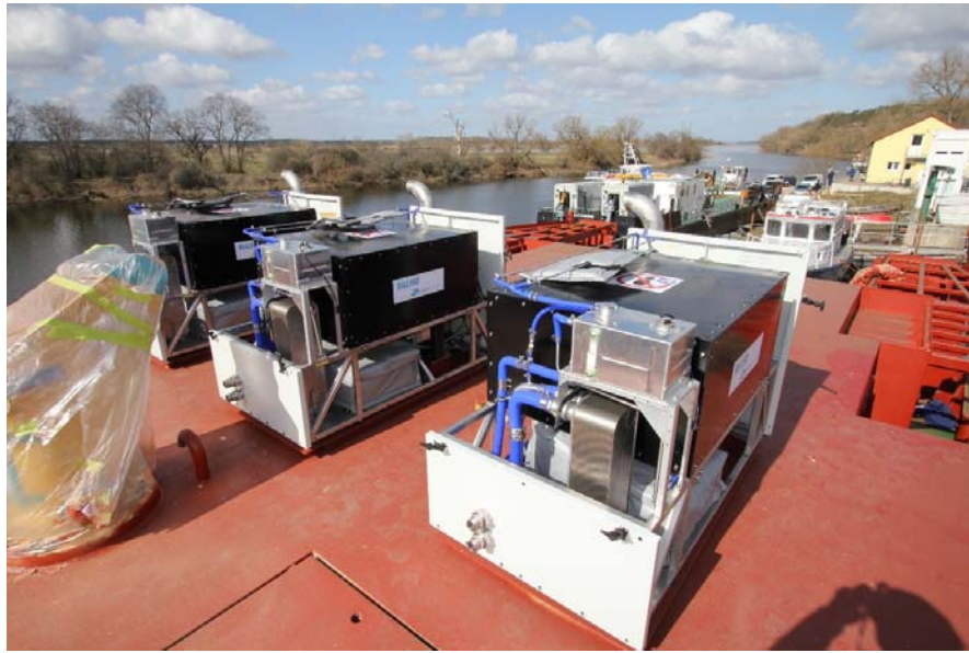
Fuell Cell Units at the weather deck
