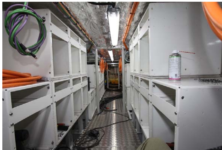
View to the Accu room (part)
