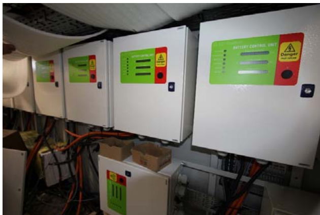
Battery Control Units (part)
